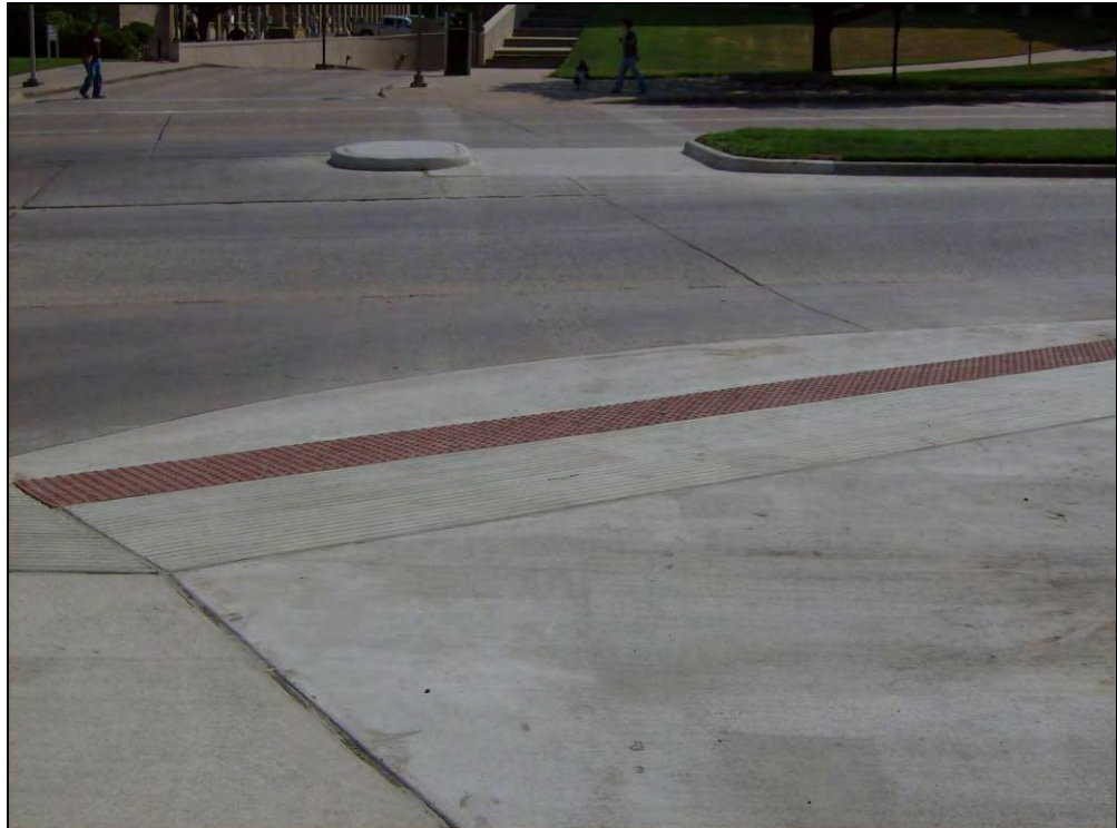
Exhibit 2. Existing curb ramp design in NE corner of N. Bizzell Street and Polo Road
